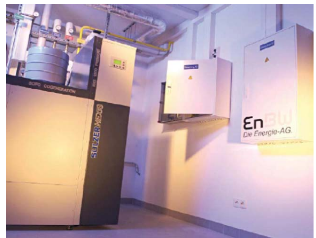
Fig. 3. Near Karlsruhe, EnBW operates a fuel cell plant in an own administration building. This was the first installation of such a plant, so we decided not to give this to a private customer but to collect the first experiences of installation and operation of a fuel cell within our facilities.
